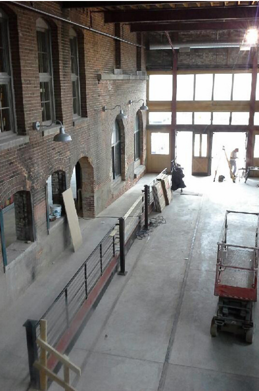
Peacock Brewery in Rockford, IL under construction (photo courtesy of Lisa DiChiera, Landmarks Illinois)
