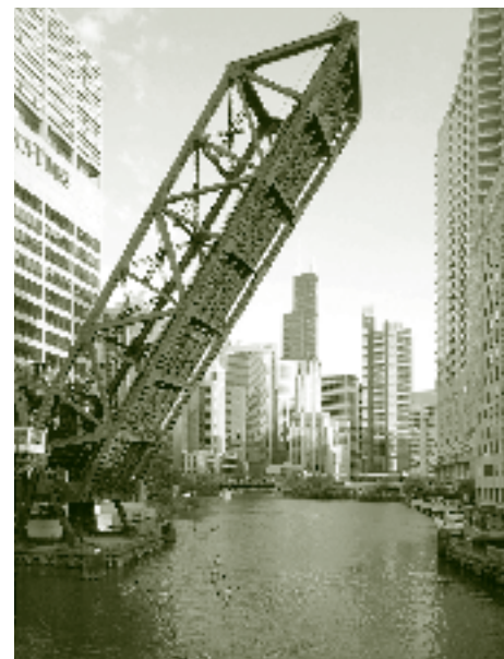
A Strauss bascule bridge built for the Chicago & North Western Railway in 1908 near Chicago's Kinzie Street. (credit: Dennis McClendon)
